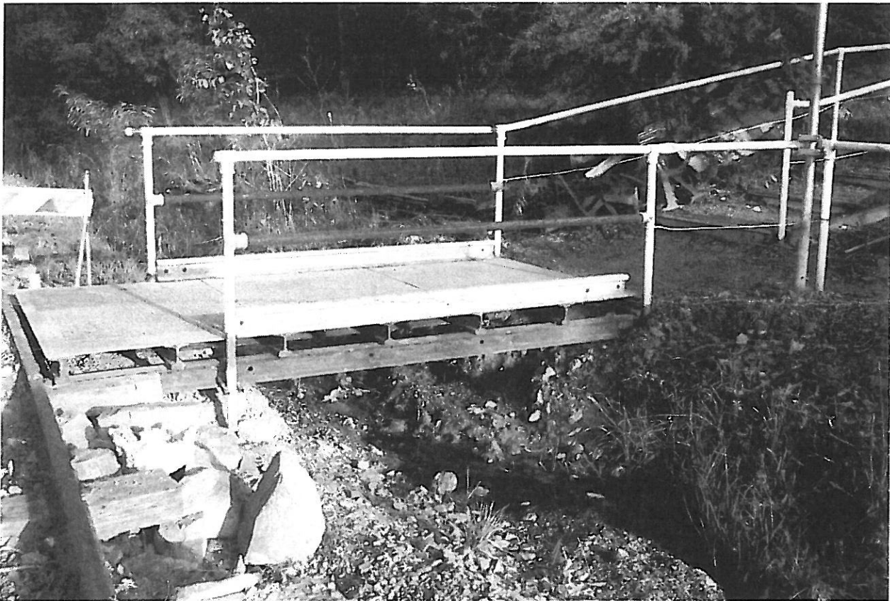
Following two torrential downpours in the Paterson area in the last twelve months, a decision was made to replace the existing earth topped piped walkway with a stronger steel and clear waterway underneath. Materials for this walkway reconstruction was kindly donated by a TRMS member.
