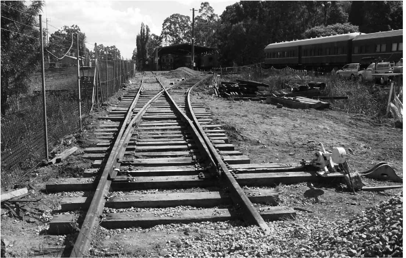
This view of the shunting neck and yard was taken on 6/12/08 before reconstruction work commenced.
