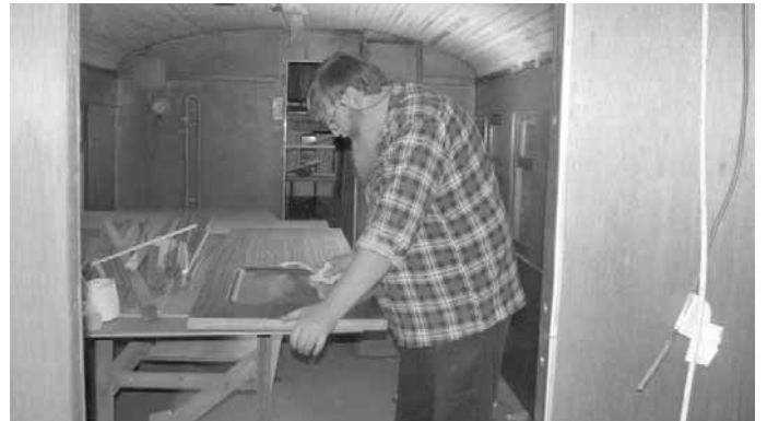
CTC 51: The restoration of the interior of CTC 51 is a slow and labour intensive task. Warren Mills is preparing an internal door for varnishing.
