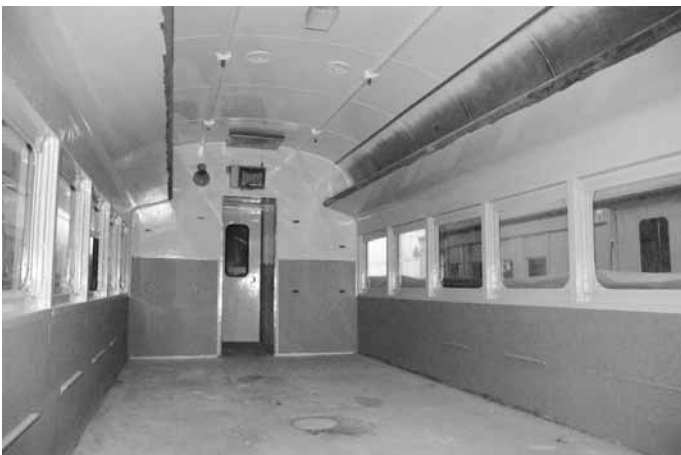
With the rotten walls painted and fittings being reinstated the interior of 729 is starting to look like a 1960's rail car again.
