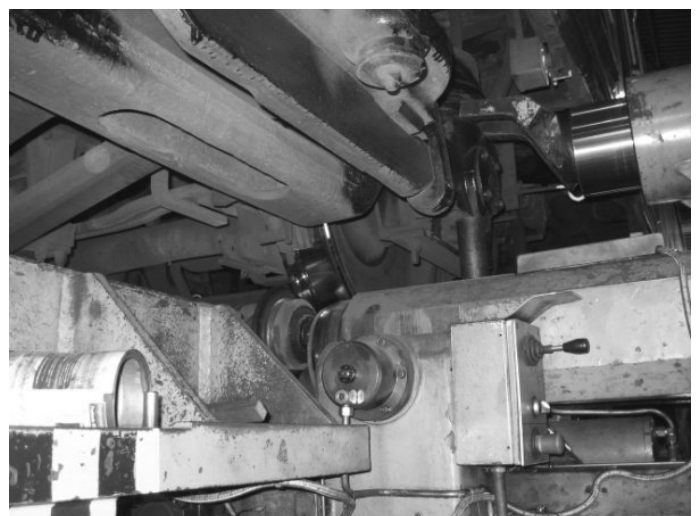
This shot taken from within the lathe pit shows the lathe equipment including mounting arrangements and an operators control position. The image of the lathe and wheel turning roller equipment reflects in the mirror like surface of the freshly turned wheel.
