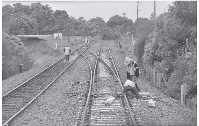
To allow the inspection train to exit the SSFL track at Enfield West the train paused for the stop block and point clips to be removed and the points wound over to set the road. This scene shows the points being re-clipped and with permission received from the Network Controller, the train commenced its journey along the MFN to Botany. Photo: Derek Rogers
