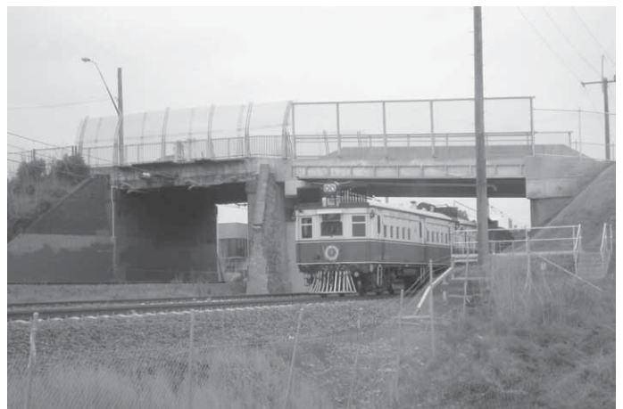
With the stop block removed, CPH's 1 and 7 are seen moving along the SSFL and disappearing under the Miller Road overbridge extension for the first time. The extent of works including bridge construction to cross over the new freight line is evident. Photo: ARTC
