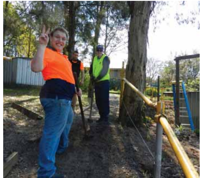
One of the many tasks undertaken by the boys was the reconstruction of the pathway and guard rail leading from the shed to the cottage following completion of the major drainage project. Photo: Stephen Davies
