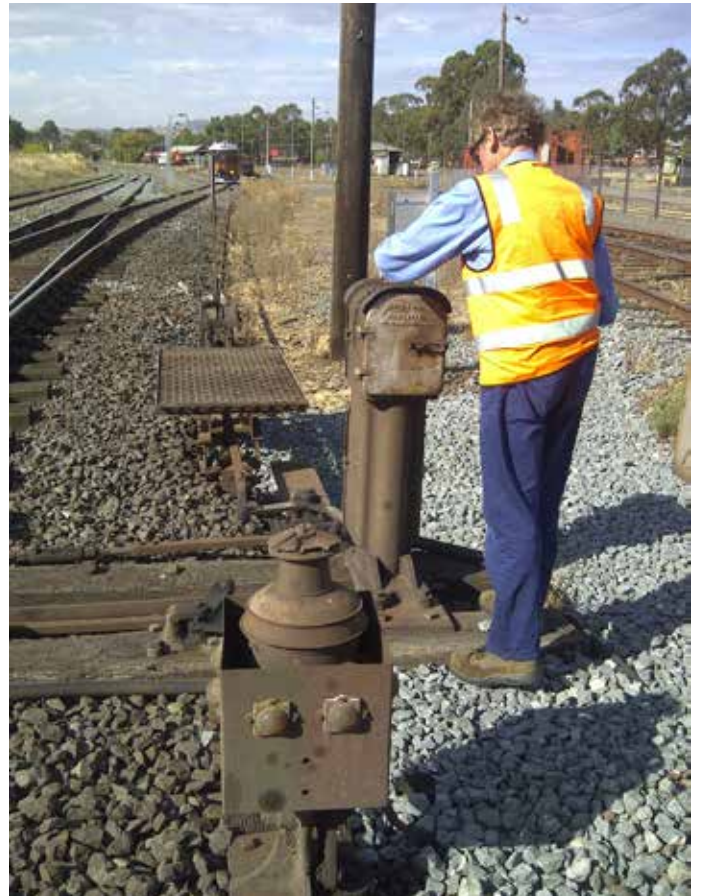
402 has moved off the ARTC mainline onto the Vline Seymour standard gauge siding. With 402 standing clear of the catchpoint Barry Dunne restores and locks the frame and electric release to normal. Photo: S. G. Preston
