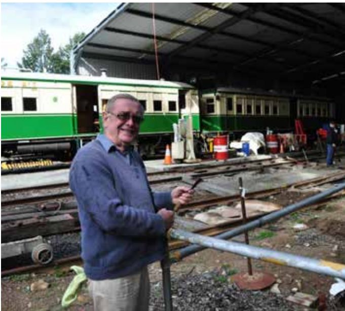
Armed with scraper and rag Jerry Jerome pauses from stripping the drain area handrails in front of the shed as he prepares to repaint the safety yellow covering. Photo: S. G. Preston
