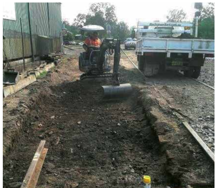
Commencement of the excavation of the Arrival Road by Gavin Bazely on 14th December 2013. Photo: Peter Kitcher
