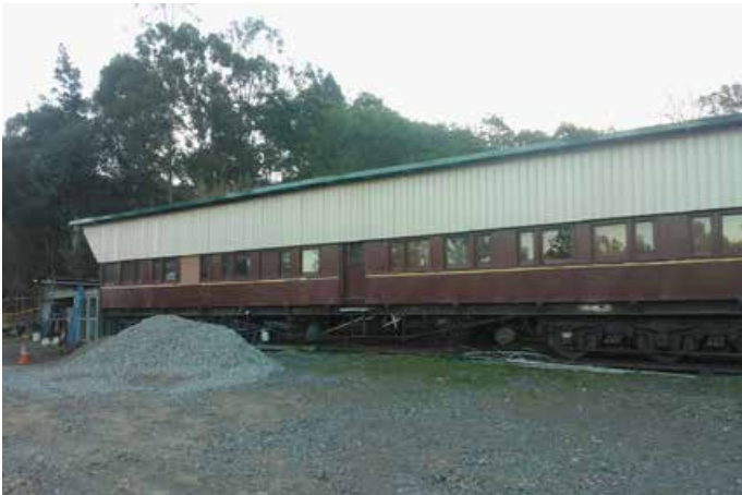
The roof cover and side protection for the TAM and BR cars is well advanced. Photo: Bruce Agland
