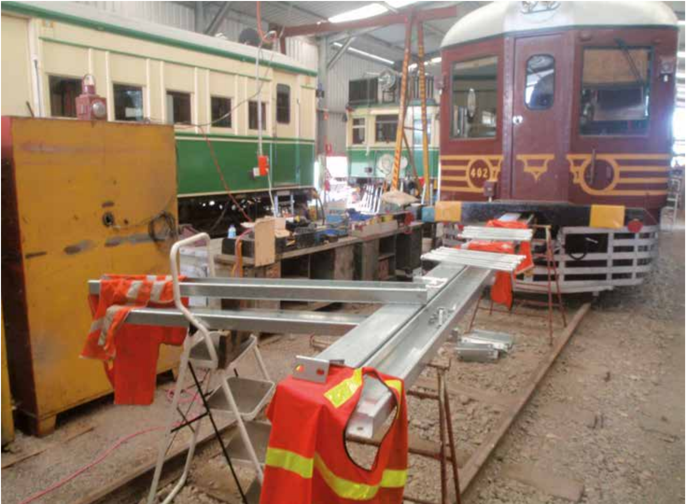
The new shed supports were first assembled inside the shed prior to erection.
