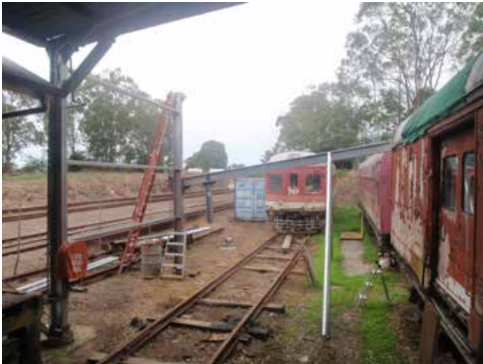
Saturday 10th January sees the rafter for the first extension bay in the process of being manually winched using chain blocks. (Photo: Bruce Kingsford)
