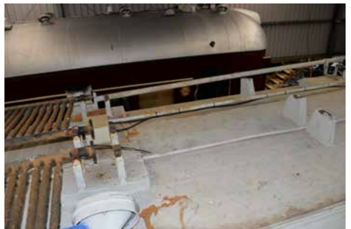
Removal of the radiator elements from 402's roof will also support maintenance and recoating of the roof structure and fittings. (Photo: SG Preston)
