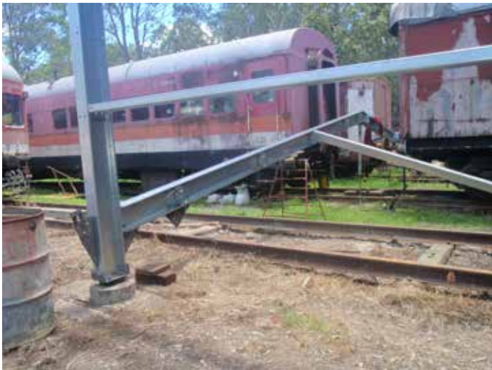
With the end rafter components bolted together on the ground preparations are in place for them to be lifted to their final position. (Photo: Bruce Kingsford)
