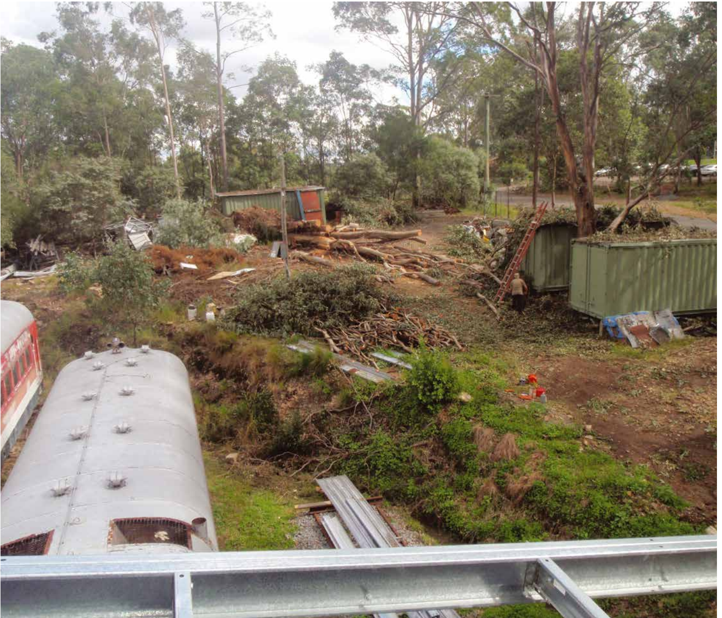
Viewed from the shed roof, the clean up and tree removal at the southern end of the depot is underway. (Photo: Bruce Kingsford)
