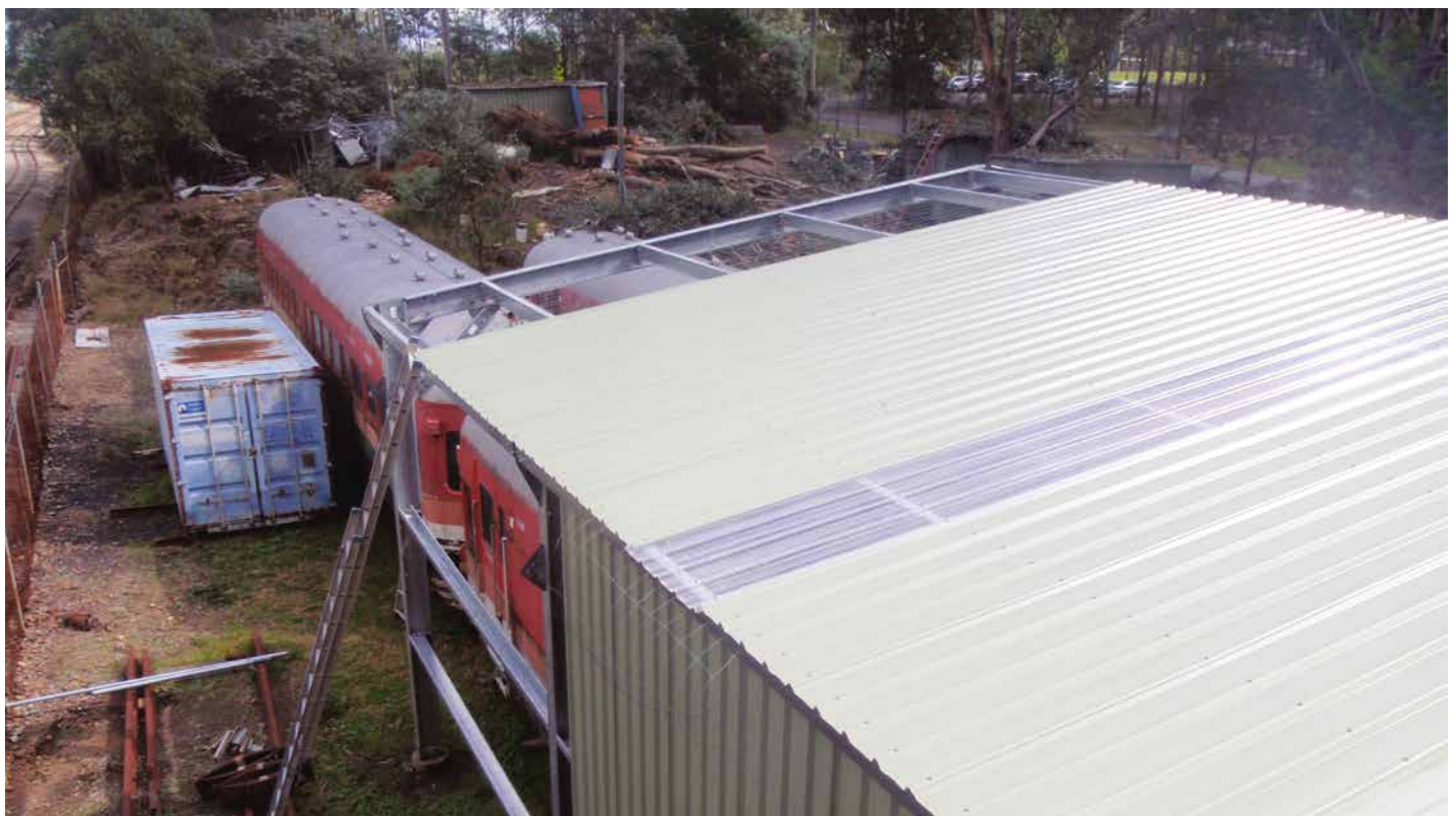
The attachment of sheeting to the roof and wall of shed extension is almost complete. (Photo: Bruce Kingsford)
