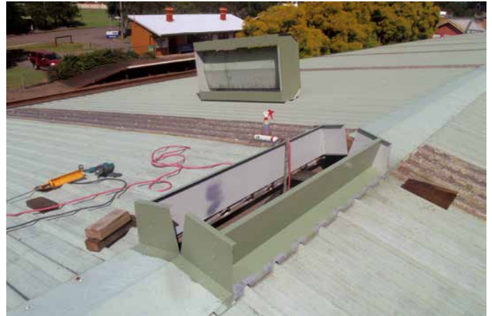
The first ridge ventilator being installed on the depot shed. These installations will improve shed conditions for operations and maintenance activities. (Photo: Bruce Kingsford)
