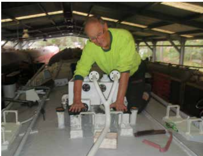
With the radiators removed for overhaul the roof fittings and other system components also received attention under the supervision of Stafford Payne.
