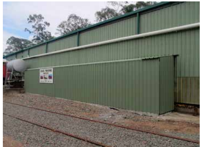
The external view of the annexe seen from the rail corridor. (Photo: Bruce Kingsford)
