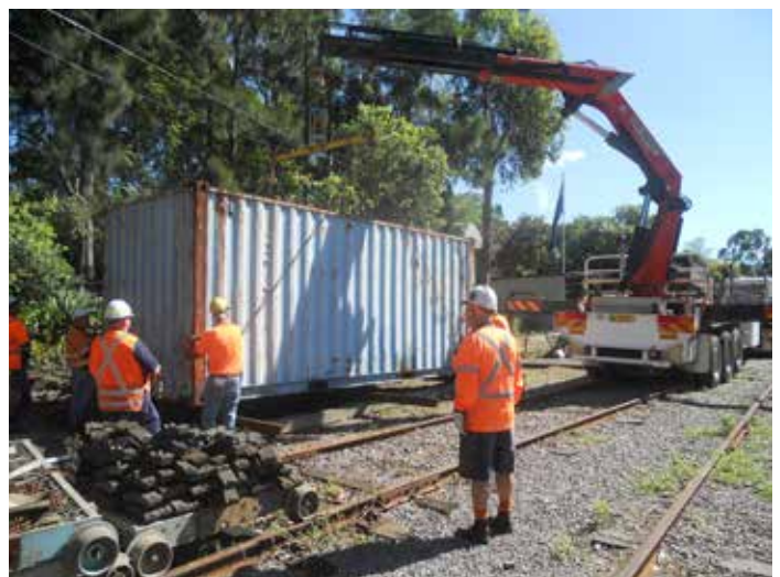
With many hands assisting and supervising, the container is moved from the end of the shed into its new position. (Photo: Rodney Short)
