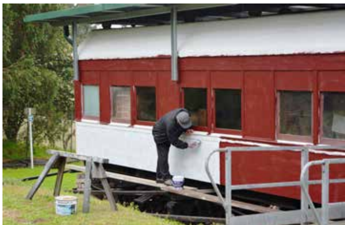
Graham Shonberg is seen applying a primer coat to the BR carriage in preparation for finalising the exterior works. (Photo: Bruce Gehrig)
