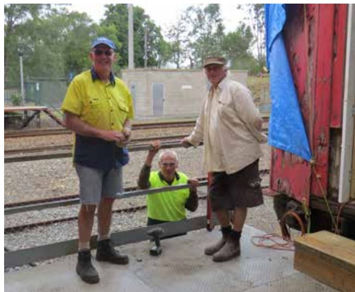
Some of the infrastructure team during building of the platform to the KB. (Photo: Mark Oxford)
