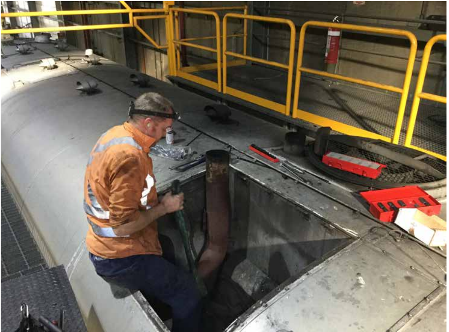
Having removed the radiator fan, Luke Wiggins fits a sling in preparation for lifting the exhaust system out in order to provide clearance to remove the radiator core. (Photo: Matt Temperley)
