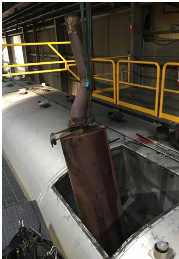
The impressive size of a 621 muffler can be seen here as it being lifted clear. (Photo: Matt Temperley)
