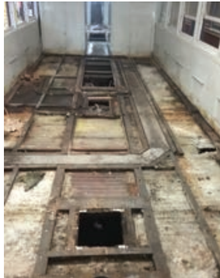
After ply removed exposing the timber frame note on the right corroded sub-floor (photo TRMS)
