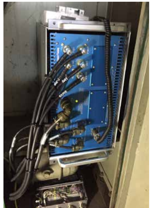
ICE radio CCU3 ancillary equipment installed into 7344. (Photo: Radio Installer)
