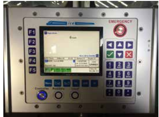
7344's newly installed ICE radio. (Photo: Radio Installer)
