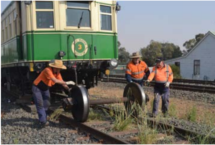
The following series of photos follow the progress of the field replacement of CPH3's axle at Gulgong. All photos by Bruce Agland. (1) Old axle out
