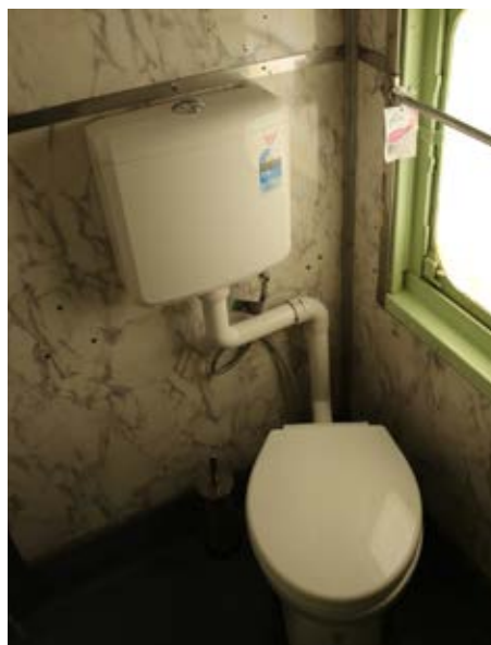
One of two new flush toilets in 721 which should finally resolve exasperating past blockage problems
