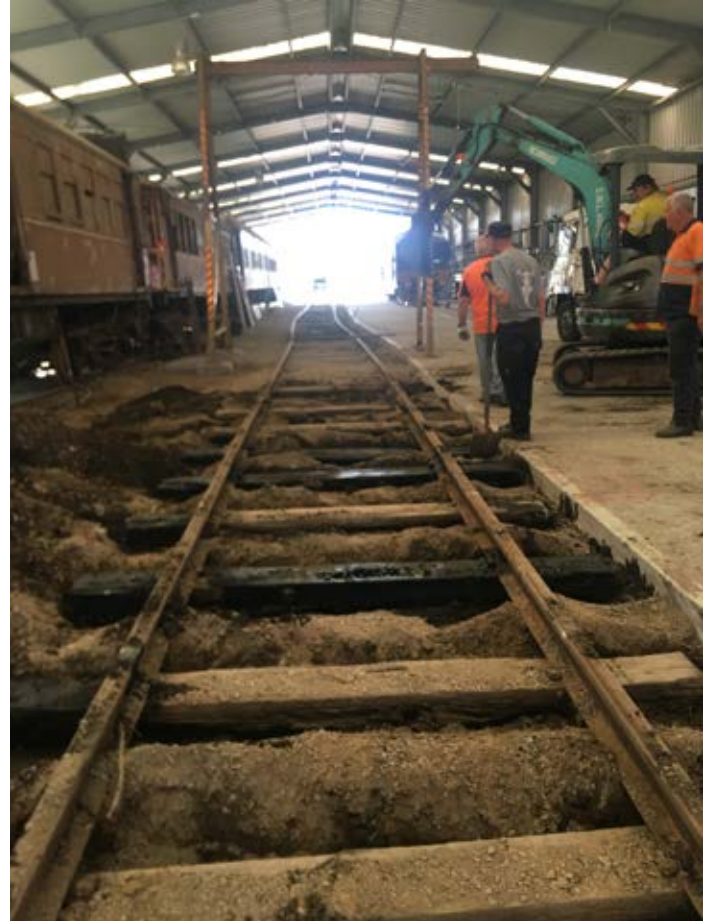
Sleeper placement has been adjusted and the track levelled in preparation to extend the concrete flooring. Photo Bruce Greenham
