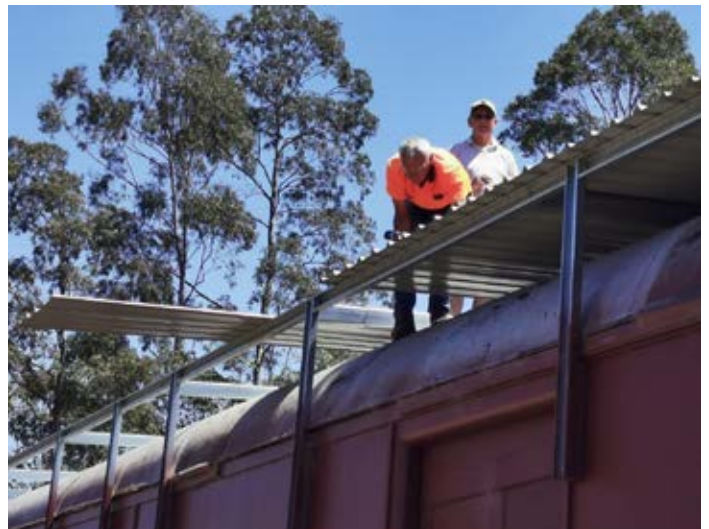
Jim Lambkin fixes new roof sheets to the canopy frame, assisted by Bruce Greenham. Photo Graeme Holloway
