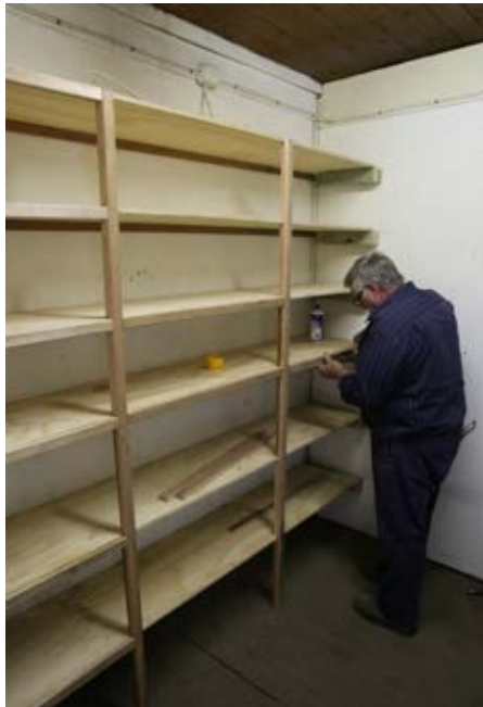
Kevin is seen here installing shelving in the electrical tools storeroom within the Goods Shed
