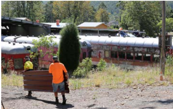
Graham and Len keep up a ready supply of new roof sheets to Jim (just visible top right)
