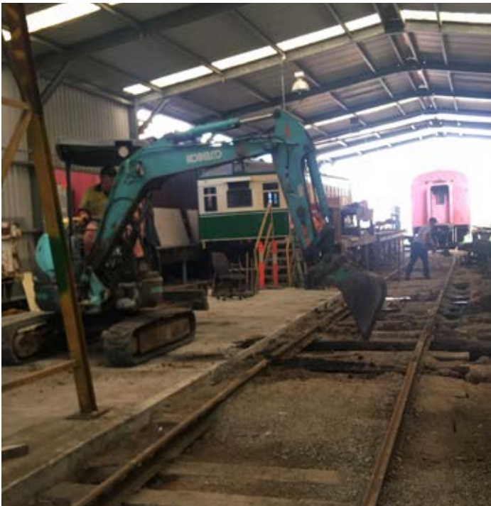
An excavator makes light work of cleaning out the rail bed next to the gantry. Photo Bruce Greenham
