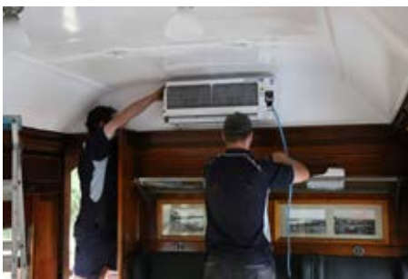
A new air-conditioner being installed in the BR lounge, and note that freshly painted ceiling
