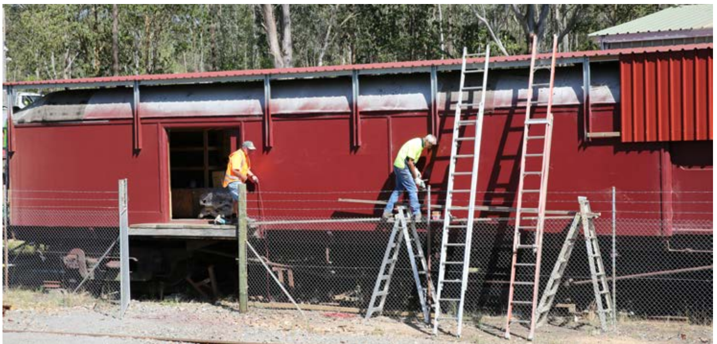
With the roof now installed Len and Jim get stuck into affixing the side wall
