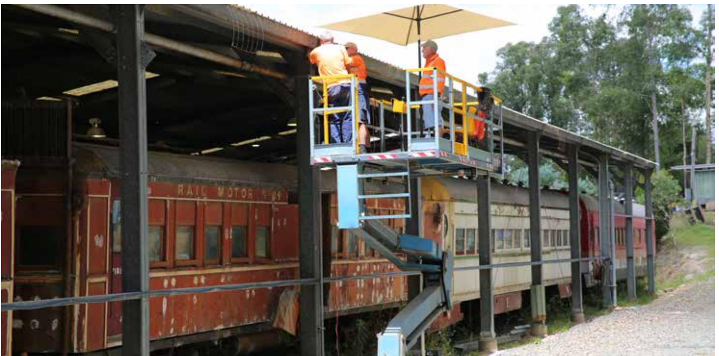
Jim Lambkin, Bruce Greenham and Len Smith make preparations to install the guttering
