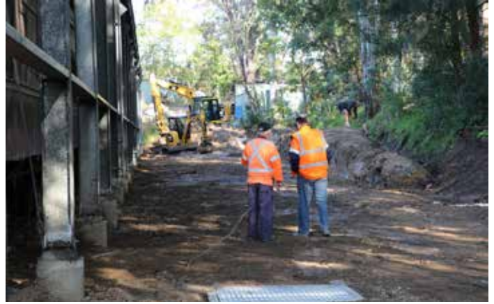
Drainage Project Manager Bruce Agland and President Arthur Burgess (left) review progress
