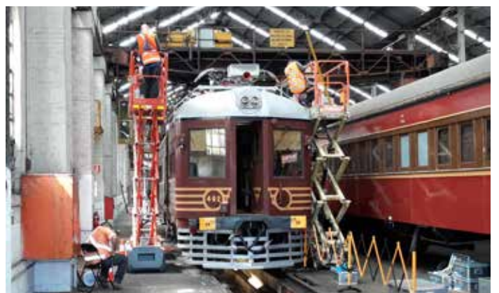
Further work on pantograph ancillaries inside the Large Erecting Shop (Bruce Agland)
