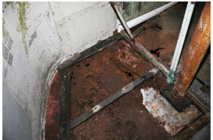
707's guards compartment and vestibule areas, showing a badly corroded metal floor, which was only discovered after the old wooden floor was lifted. The metal floor was later replaced.
