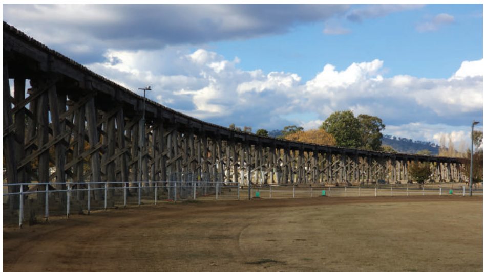
At Manilla, a stop was made to photograph the magnificent curved viaduct over the Namoi River flood plain. Captured on 12 Jun 2023, most of this structure is about to be removed due to safety concerns
