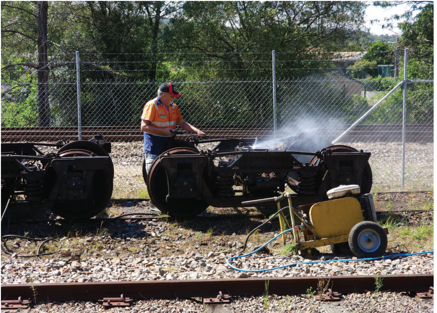
Using a high-pressure water jet, Allan Beard removes many years of grime from bogies recovered from CPH 7, on 29 Nov 2023. These will be the next set to be overhauled.
