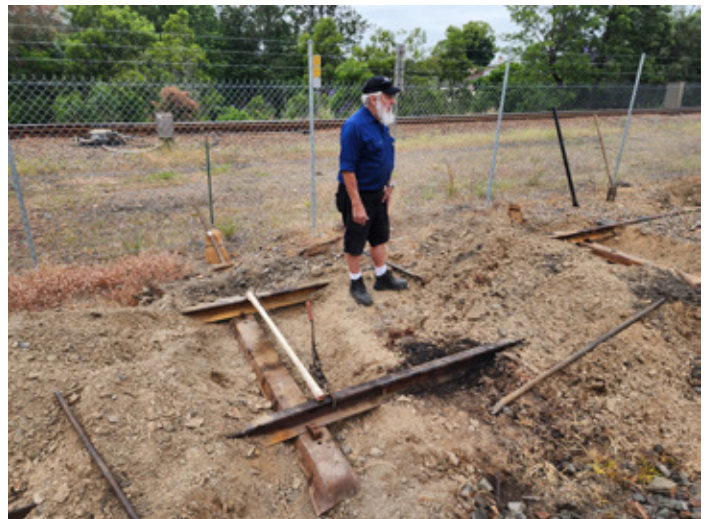
Condemned wooden sleepers have been removed and replaced with steel sleepers, 6 Nov 2024.
