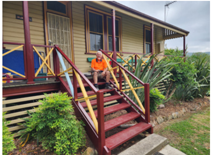
Tony Price has replaced the side veranda, railing, and steps on the former Station Masters Cottage. Seen here on 6 Nov 2024, he has just one diagonal brace left to paint.
