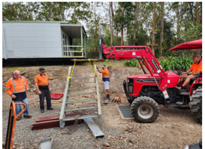
New steps are lifted into position. These will provide access to the new demountable meal room. 6 Nov 2024.
