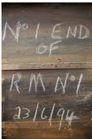
The date of prior work activity on CPH 1, revealed behind the cladding, once more sees the light of day. [TRMS]
