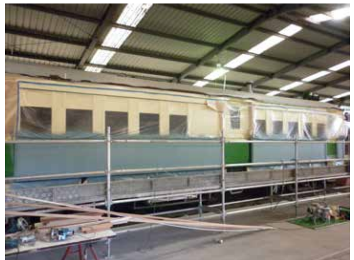
New cladding has been fitted to CPH 1 and it is seen here masked up ready for the side panels to be painted in distinctive Emerald Green. [TRMS]
