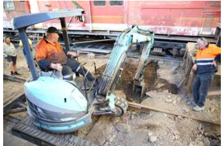
An excavator makes light work of digging a trench in the Main Shed in preparation for drainage works, watched on by Peter Macfarlane. [TRMS]
