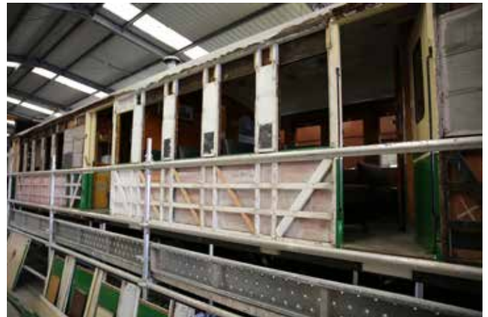
Using 'S3' grant funding, CHP 1 undergoes external remediation. It is seen here with its windows and outside cladding removed, revealing the wooden frame. [TRMS]
