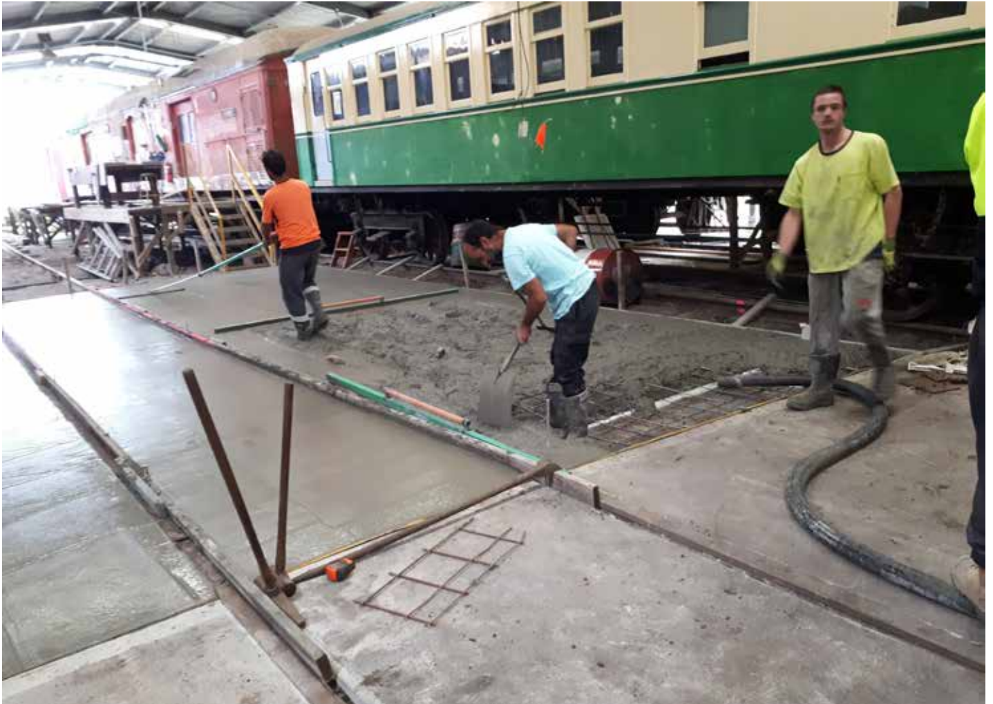
The concrete pour is nearly complete and the surface is being finished off. [TRMS]
