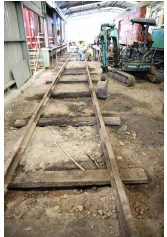
The No.1 road is cleaned out and the sleepers have been dislodged to enable the rails to be levelled before being set in concrete. [TRMS]
