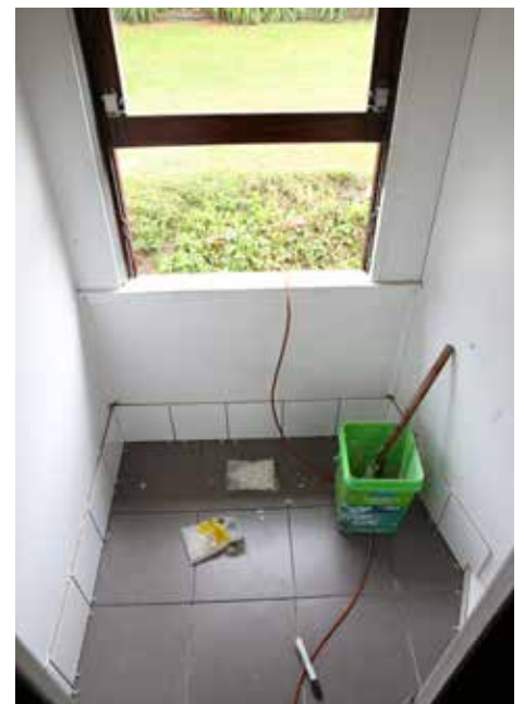
New tiling has just been laid in the TAM lavatory compartment prior to the installation of a new flush toilet. [TRMS]
