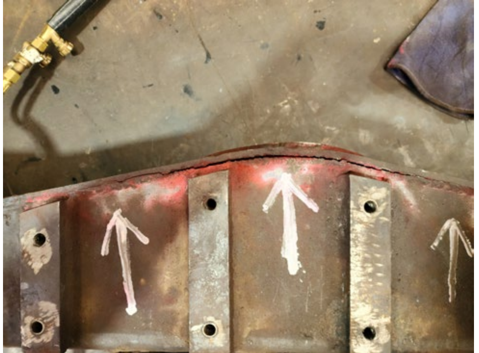
A fabricated component on the bogie bolster showing failure of the weld seen before repair by our boilermakers
