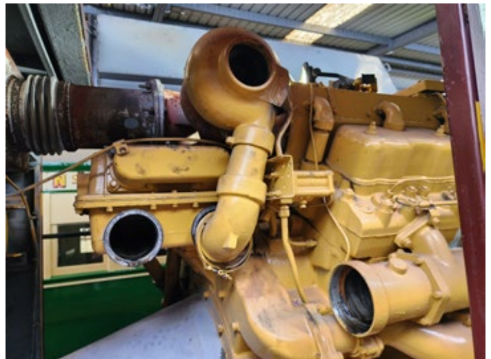
Loco 7344 engine, showing one of two turbochargers that needed replacing, still to be removed and connected to the aftercooler, also later removed for cleaning.
