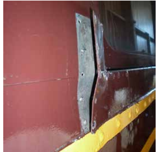
A plate has lifted near a window corner and rivets have been pulled clean out.
