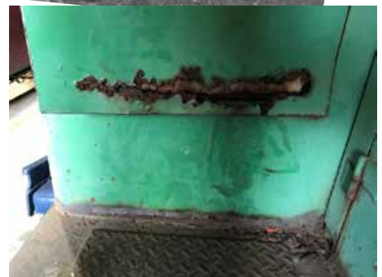
Top: An example of rust in a canopy door.
