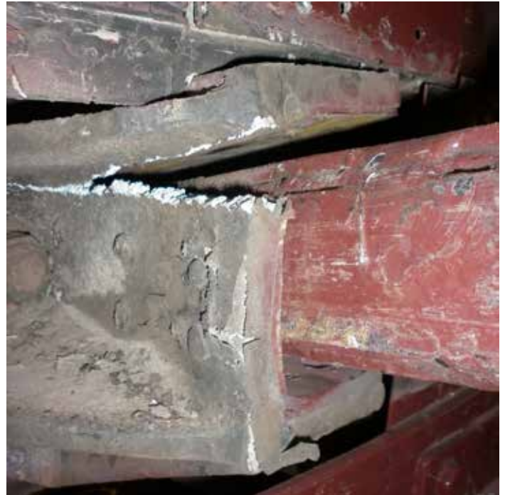
The damaged plunger bar guide and bent plunger bar (behind the front buffer beam).
