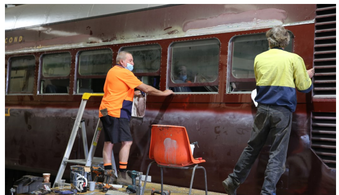
Graeme and Noel attach new side cladding around the window frames of 621
