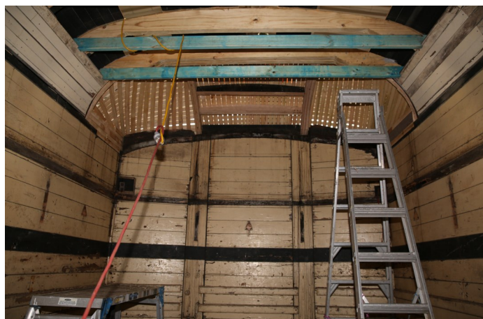
The interior of the MHO showing new curved roof end under construction, 20 Mar
