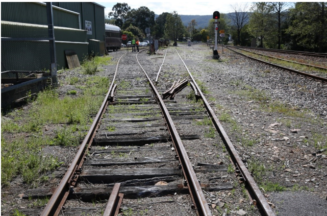
Abandoned siding outside our Depot fence. Photo: Robert Spencer
