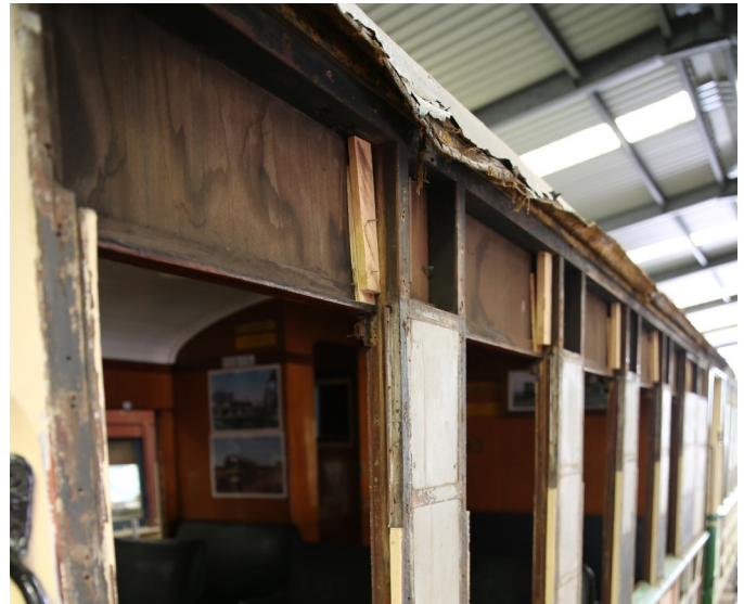
CPH 1 roof cladding was found to be in poor condition. Photo: Robert Spencer
