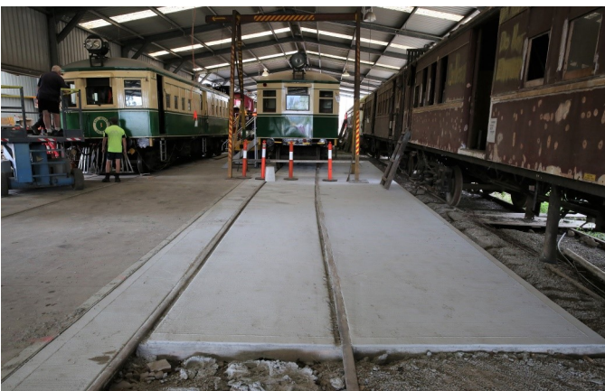
Newly poured concrete on No. 2 Road. In the background Paul Horder (just visible) removes marker lights and other electrical components from CPH 1, watched by Glen who will repair the body ends.
