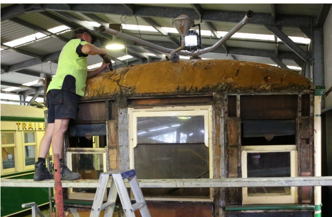
Glen Davies strips back the roof covering from the rear of CPH 1
