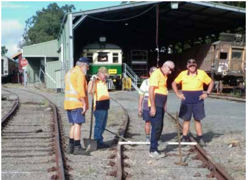
ABOVE: Jim Lambkin and fellow volunteers carry out repairs at the site of the derailment, 16 Mar 2022
