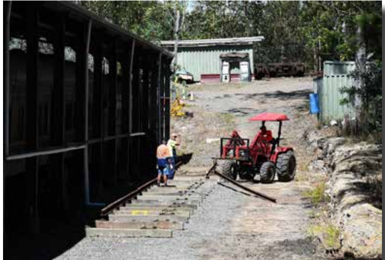
After COVID delays and months of wet weather, work finally gets underway on the 4th Road, 3 Nov 2021
